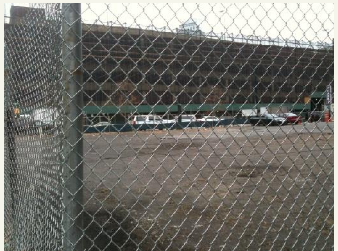
Looking north from Bond Street to Schermerhorn Street. The parking lot is being demolished to accommodate constructions of 700+ units with ground floor retail.
